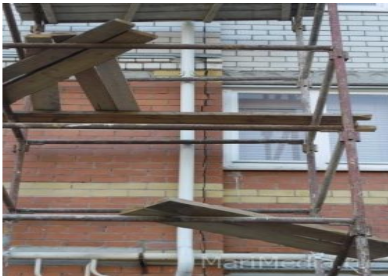
Figure 1. Defects of the investigated building
